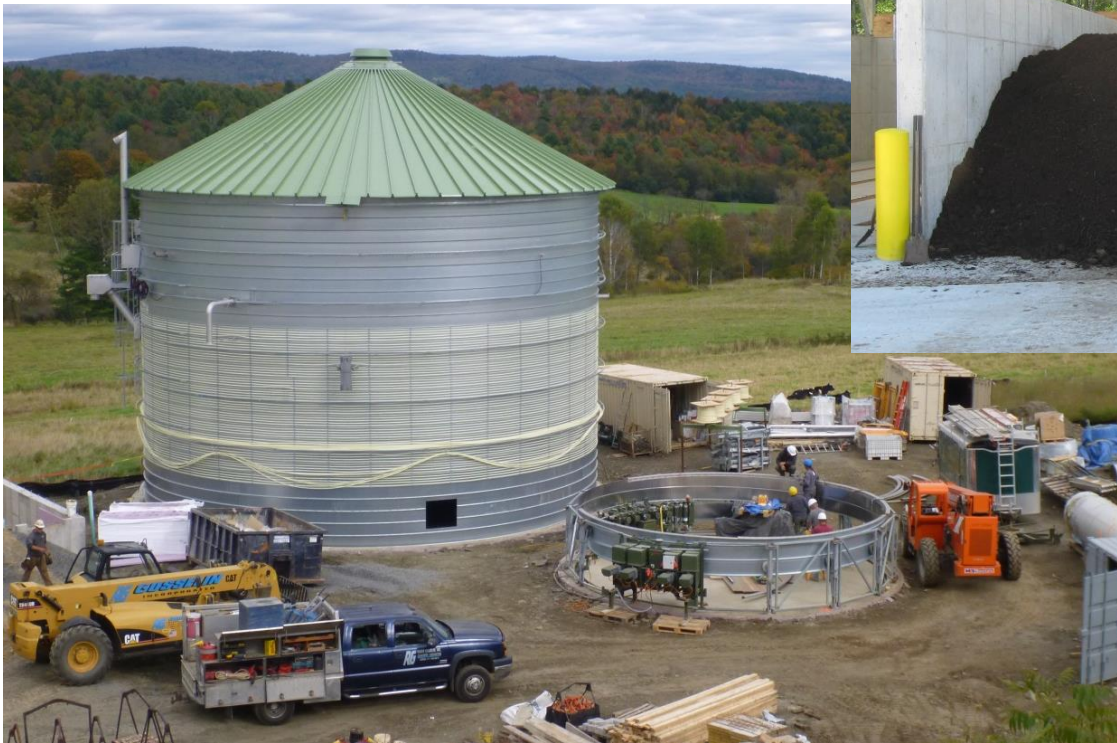
Vermont Technical College's Anaerobic Digester
